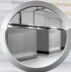
陈旧的空气压缩系统 带来高昂的能源损耗 Old compressed air system High energy consumption
